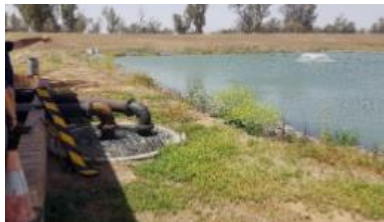
Gunnedah STP Maturation Pond
