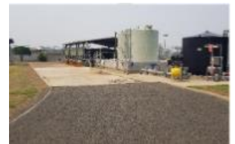
Westdale STP (Tamworth Regional Council) Chlorine dosing unit
